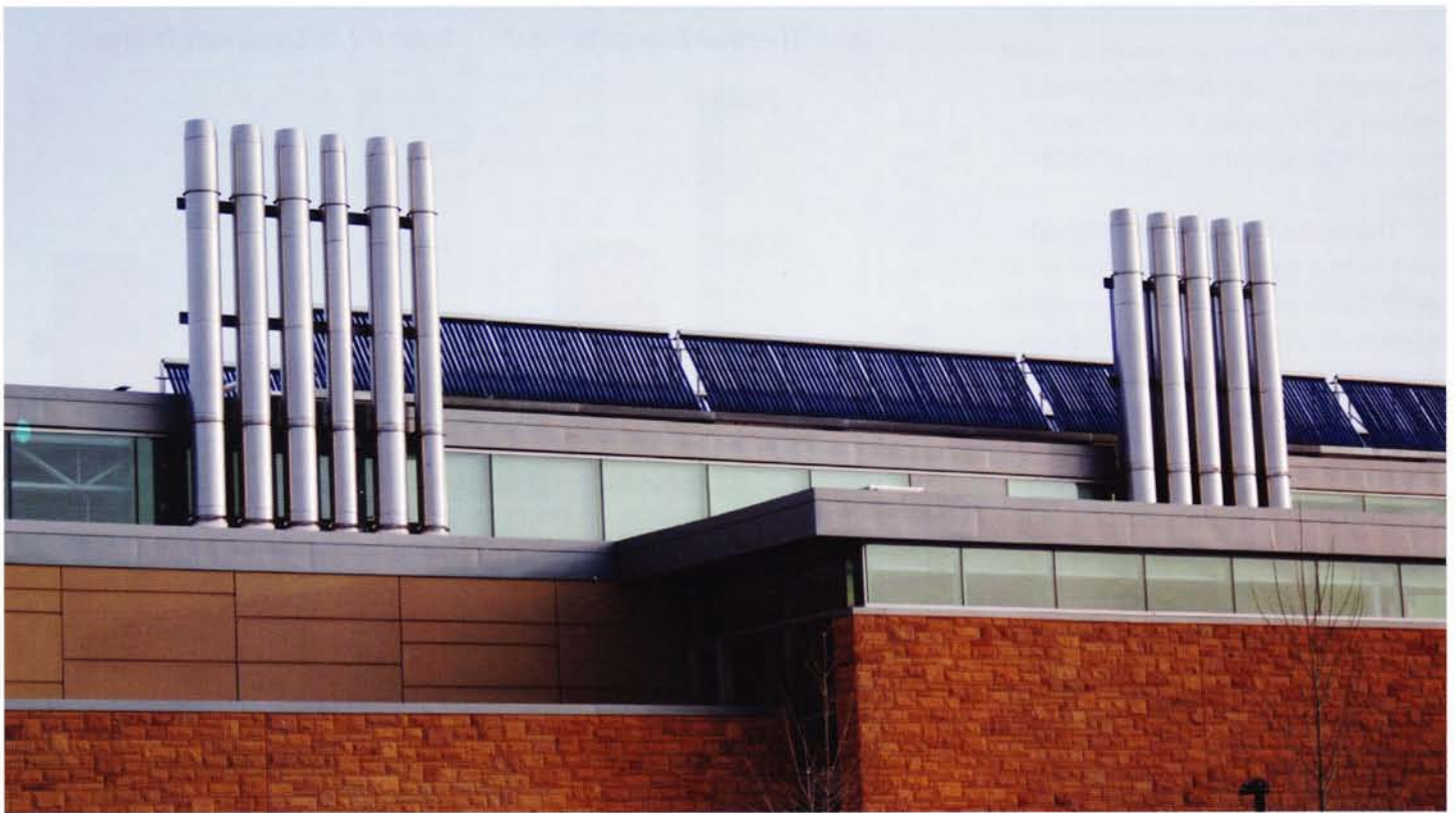
Solar thermal "evacuated tube" heating system on the roof of the UW Visual Arts Building. These active solar systems are an integral part of the aesthetic design and are not perceived as an eye-sore by most.
