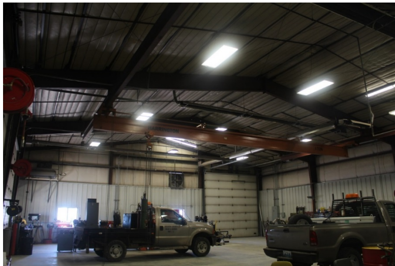
Figure 21. Goshen County Road and Bridge shop interior, Torrington, post lighting retrofit
