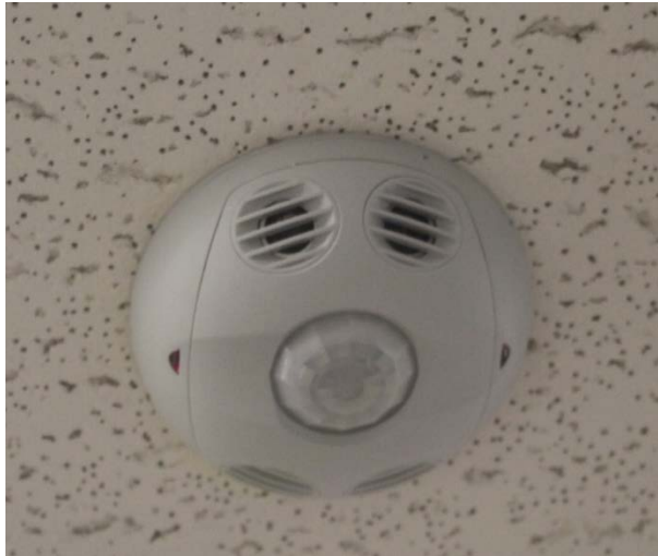
Figure 11. Goshen County Extension Office, Torrington, ceiling mounted occupancy sensor
