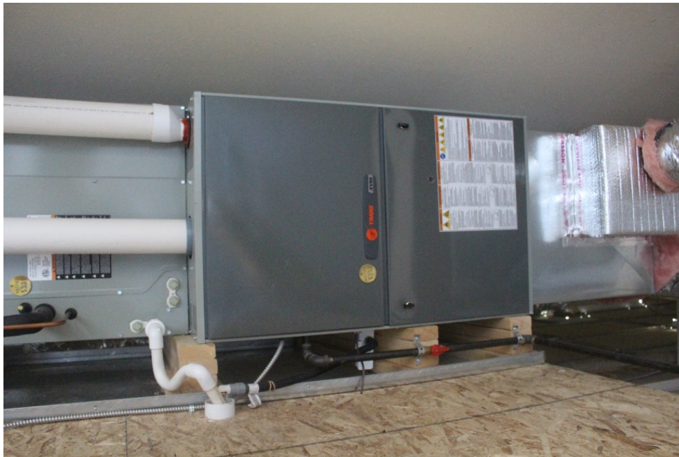
Figure 9. Goshen County Extension Office, Torrington, after HVAC upgrade
