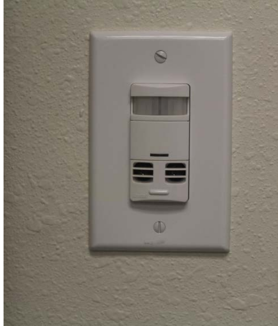
Figure 10. Goshen County Extension Office, Torrington, wall-mounted occupancy sensor
