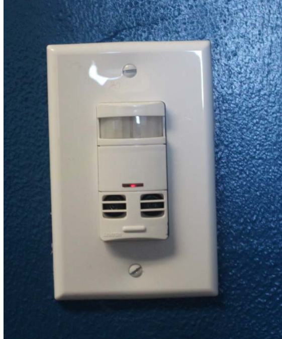
Figure 22. Goshen County Road and Bridge office, Torrington, wall-mounted occupancy sensor
