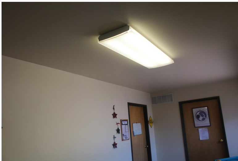
Figure 18. Goshen County Public Health interior, Torrington, lighting post-retrofit
